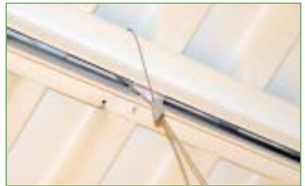
Cable strung over a ceiling joist is one method of supporting fabric duct.
