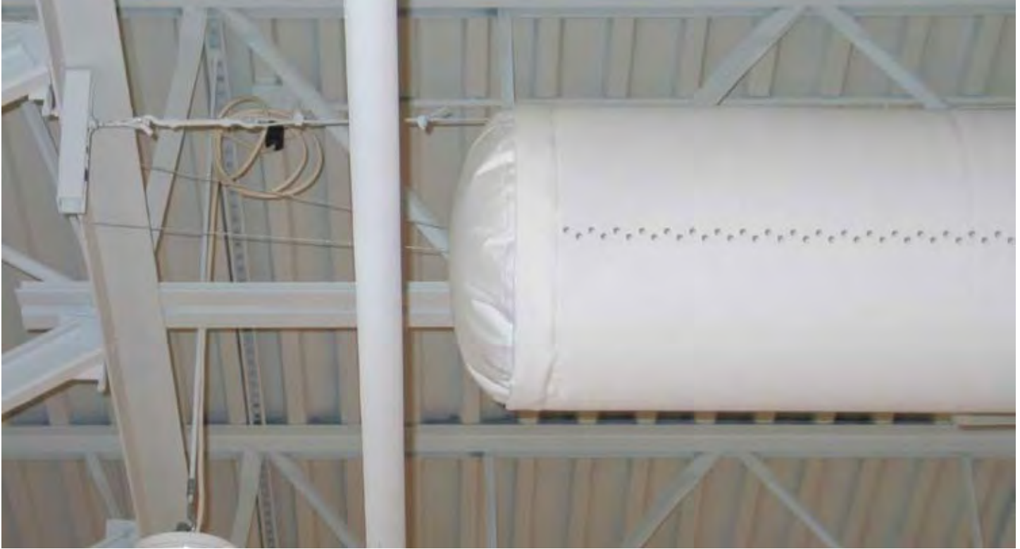
Nike Interior Fabric ductwork not only eliminates using metal resources, but the linear diffusers that run the entire length of the duct produce a more even airflow. This limits mechanical equipment runtime—thus saving energy and operation expenses. | Photo: DuctSox Corp., Dubuque, Iowa.
