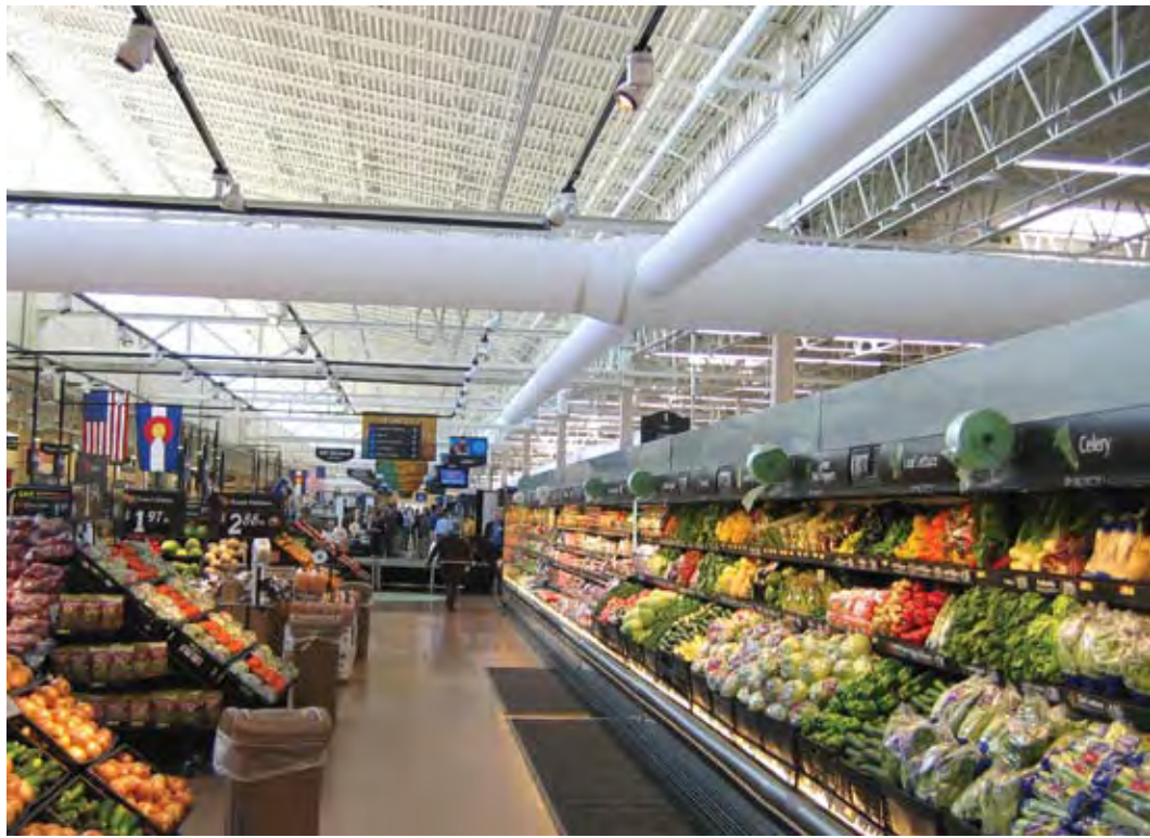
Store designers, architects and retail engineering departments at retailers such as Wal-Mart are taking the lead in focusing on green design HVAC systems. They are experimenting in new stores with higher efficiency mechanical systems and fabric duct air dispersion systems instead of metal duct, such as in this Wal-Mart in Aurora, Colo. | Photo: DuctSox Corp., Dubuque, Iowa.
